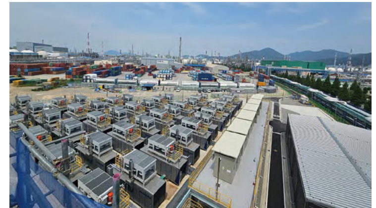
▲ Yeosu Hydrogen Fuel Cell Power Plant
