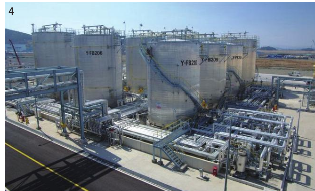
3. Metallocene Lab 4. Polybutene Storage Tanks at the Yeosu Production Facilities
